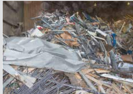
Materials from demolitions are sorted for resale/reuse while municipal waste is simply moved to the back for transfer to area landfills.
