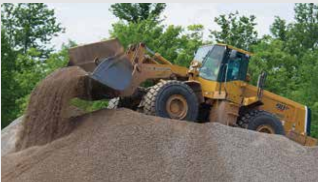
Smaller Kawasaki (KCM) loaders are used to load dump trucks and manage the piles of crushed material.
